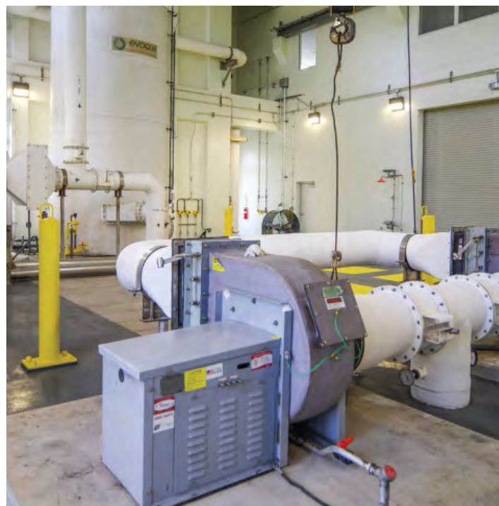
► City of Sarasota - Lift Station No.87
