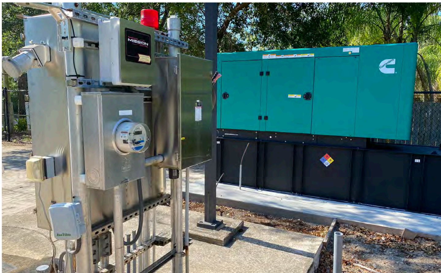
► City of Palm Coast - Backup Power for 30 Generators
