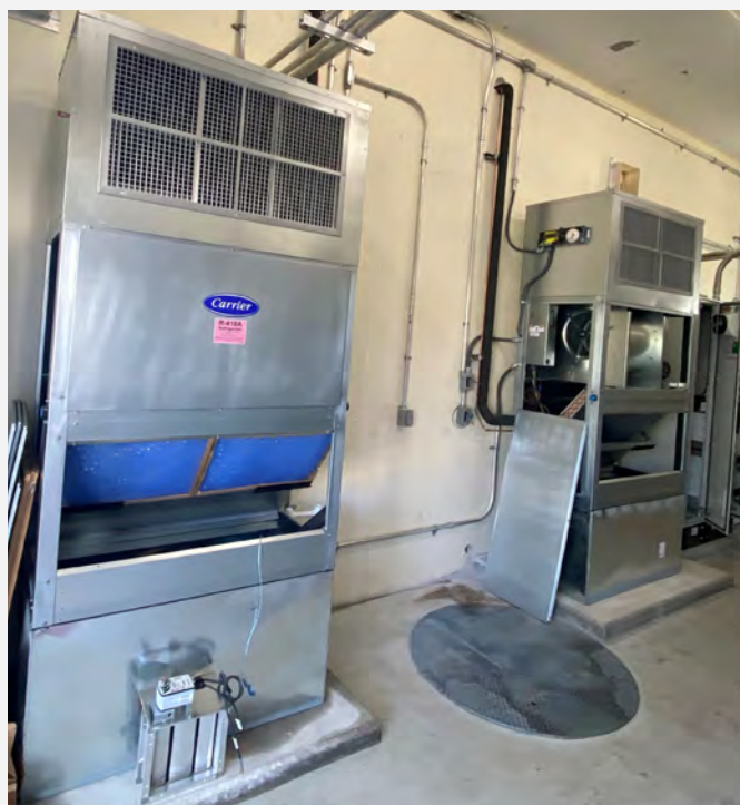
New redundant air handler units designed by Carollo with features to control humidity in electrical rooms and increase electrical equipment reliability.
