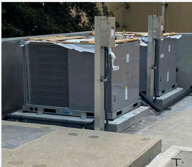
Redundant air conditioning units designed by Carollo.
