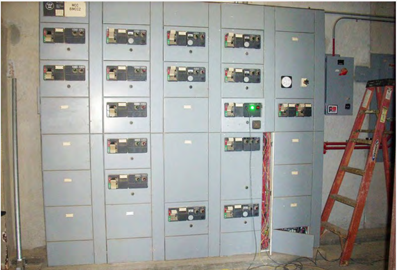
MCC at Dewatering Building is in need of upgrades.
