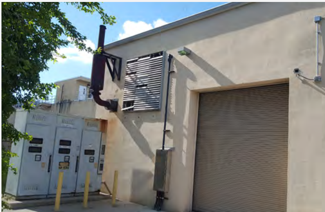
Exterior 5-kV switches to be removed.
