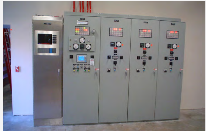
Example of separate low-voltage control cabinets for synchronizing generators.
