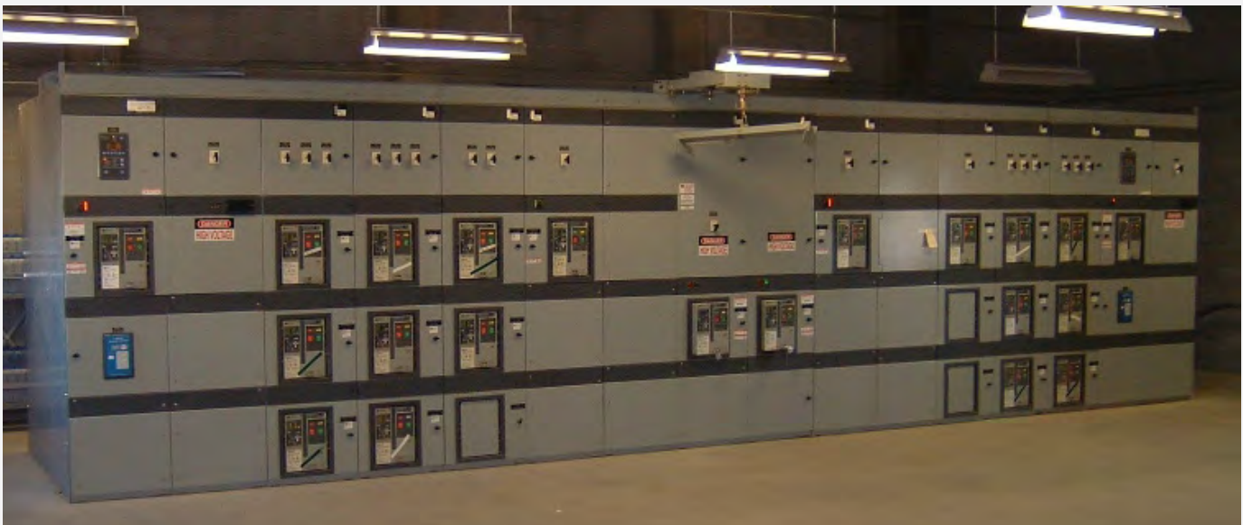
Example of a 480-v switchgear design with a center tie-breaker to provide redundancy.
