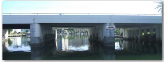
Hardesty & Hanover provided CEI services and remedial design services for the Pine Tree Drive Bridge rehabilitation project.
