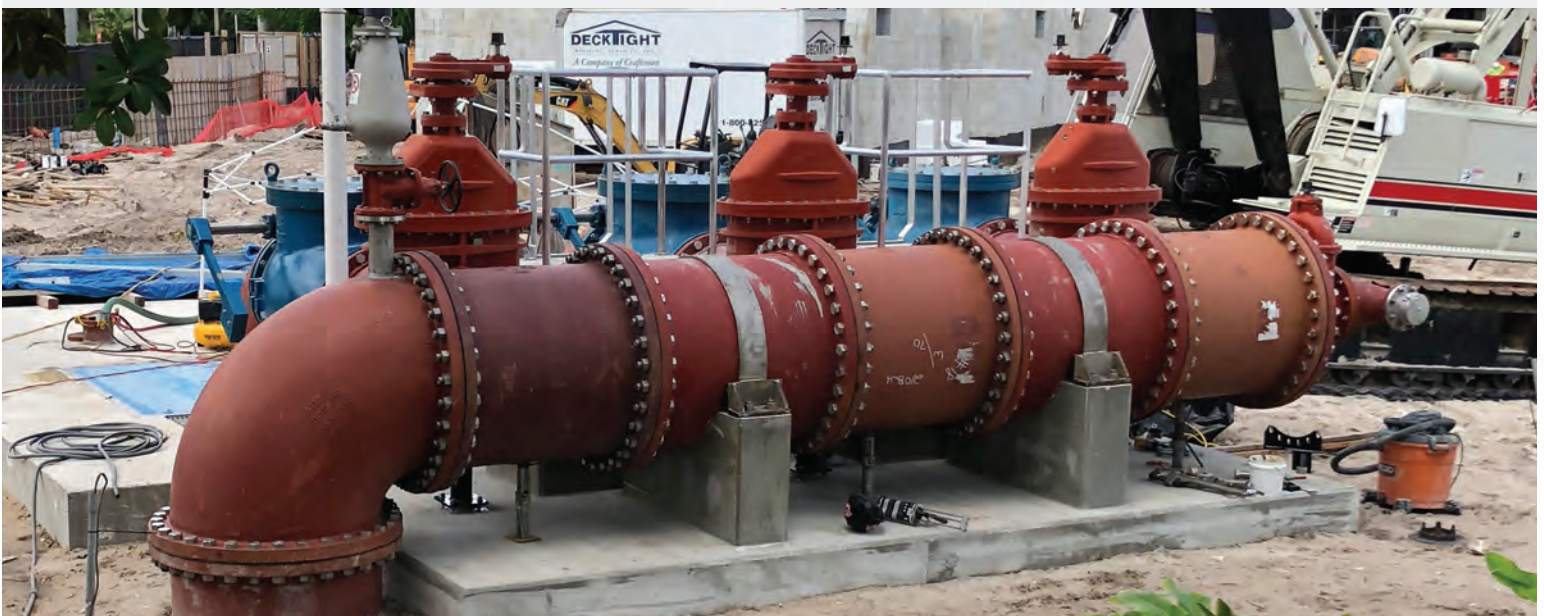
HARD ROCK HOTEL MASTER LIFT STATION 36" DISCHARGE PIPING
