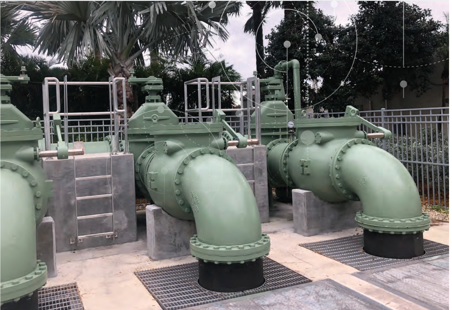
HARD ROCK HOTEL MASTER LIFT STATION MECHANICAL PIPING
