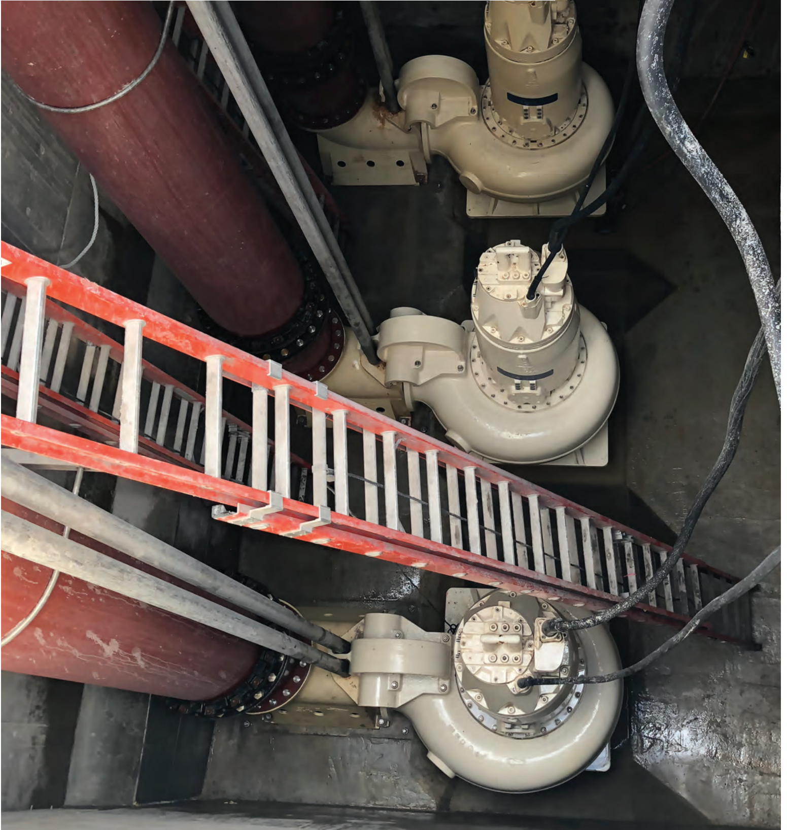
HARD ROCK HOTEL MASTER LIFT STATION (3) 135 HP FLYGT PUMP INSTALLATION
