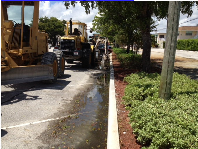
Existing drainage issues along NE 1 st Street
