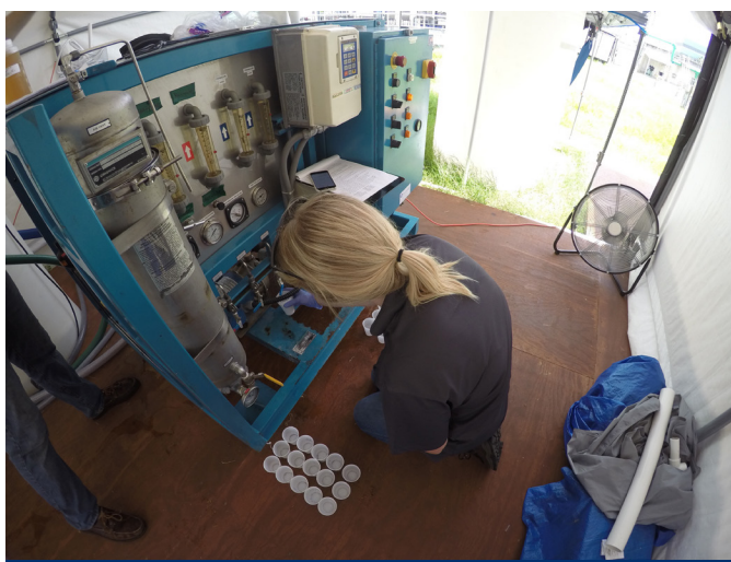
Tetra Tech Engineer Adjusting Treatment at Hillsborough County's Pilot DPR Project
