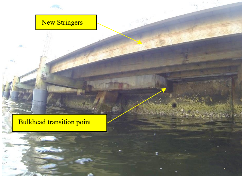
Plate O View beneath dock at bulkhead transition point Note repaired section of timber dock
