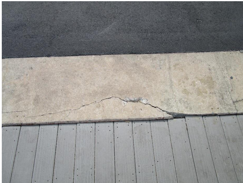
Plate L Significant cracks in concrete cap
