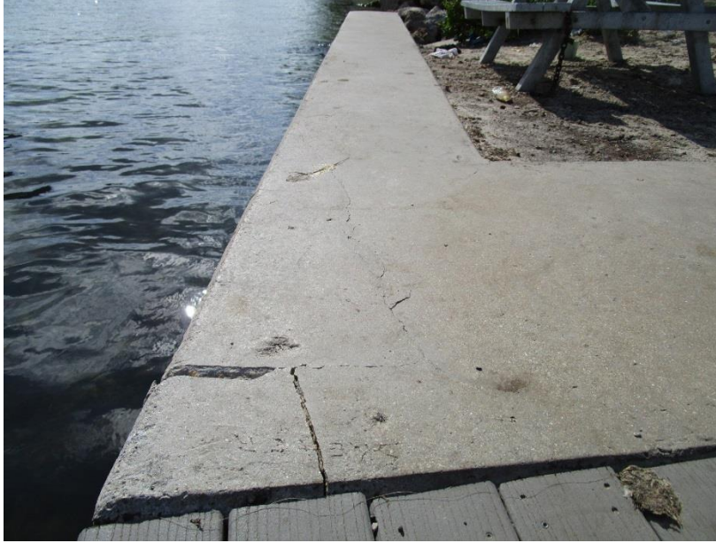
Plate A South View at East End along ICWW Note major crack at corner
