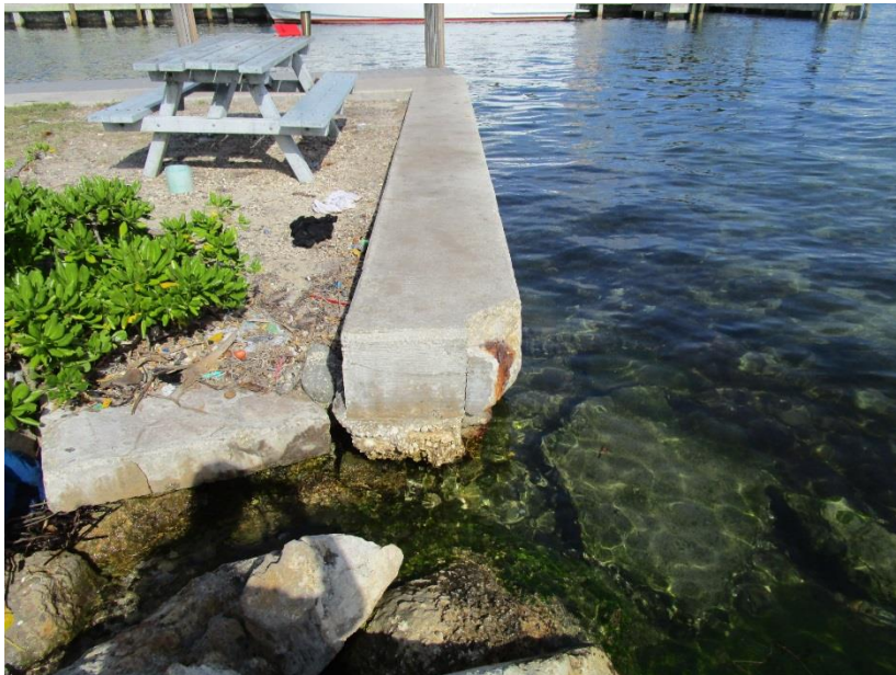
Plate D North View at East End along ICWW. Major crack / loss of concrete and spalling corner.
