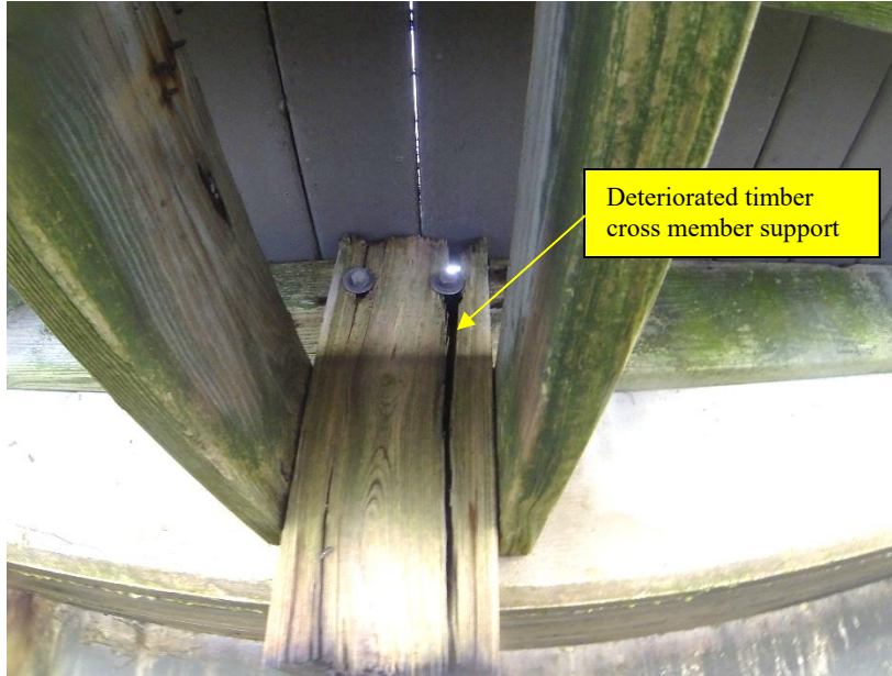
Plate I Cracked / deteriorated timber cross member support
