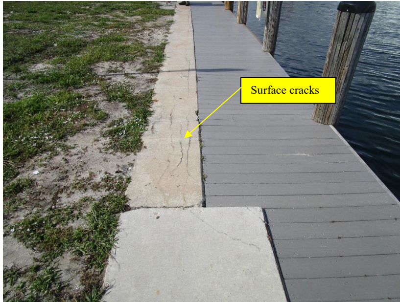
Plate K West view at transition from repaired bulkhead section to original bulkhead structure
