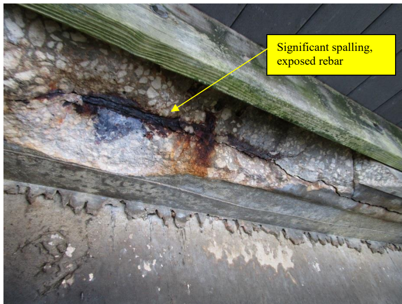
Plate R Typical condition of bulkhead cap
