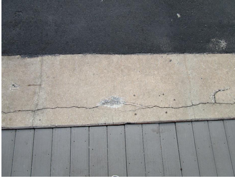
Plate M Significant cracks in concrete cap
