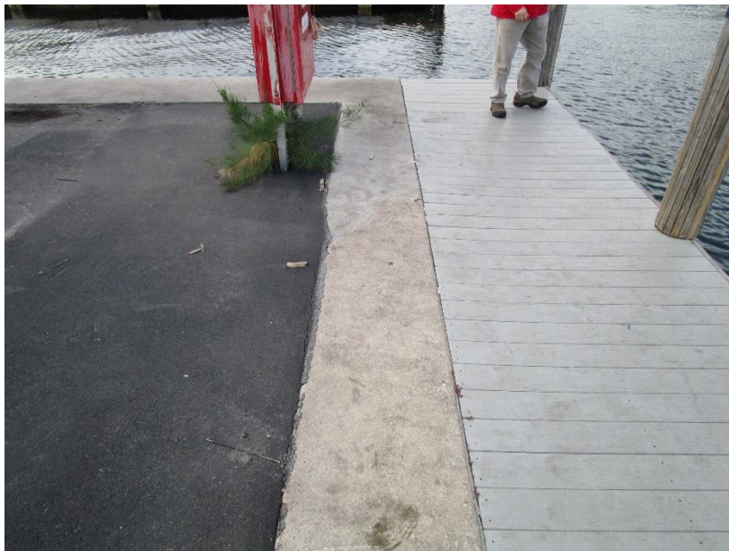
Plate N West end of bulkhead under current assessment
