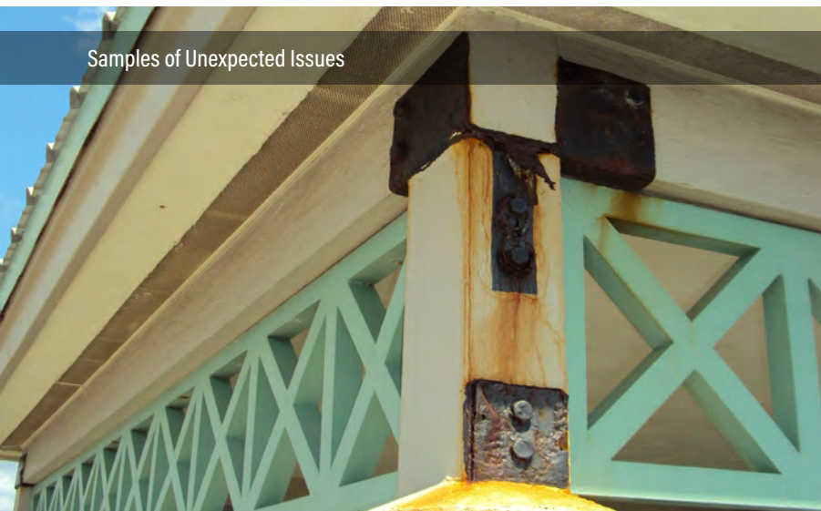
Discovery of a missing steel connection during routine inspection for a beach pavilion.
