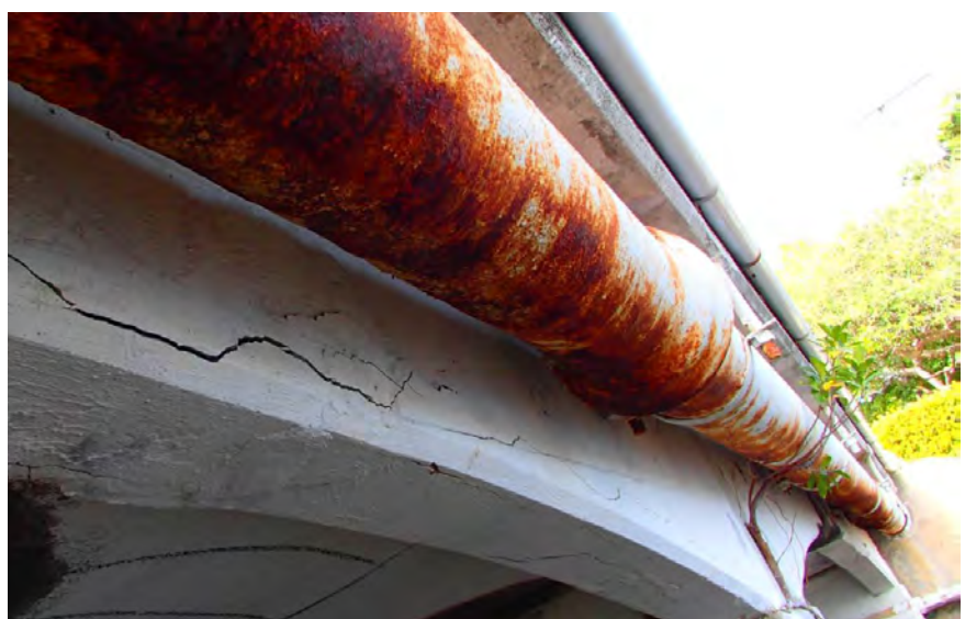
Discovery of bridge structural failure following a satisfactory rating by FDOT.
