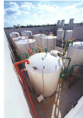
Sulfuric acid and scale inhibitor have been industry standard chemicals for pretreatment.
