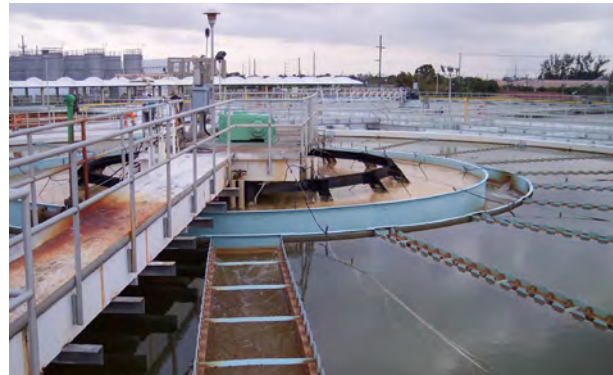
Detailed performance evaluations of Miami-Dade's 165-mgd of SCCs (accelerators similar to Pompano Beach) were conducted by Carollo.
