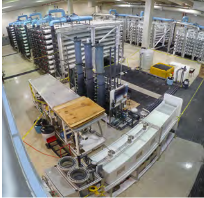
Carollo pilot tested a cost-effective approach for RO concentrate recovery in South Florida.
