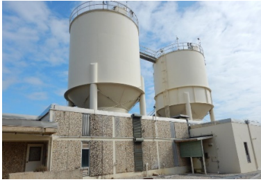
Lime Slaker Units
