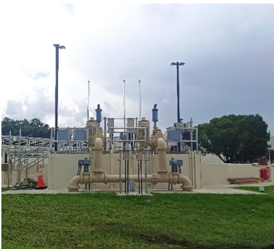
Basin Pump Station
