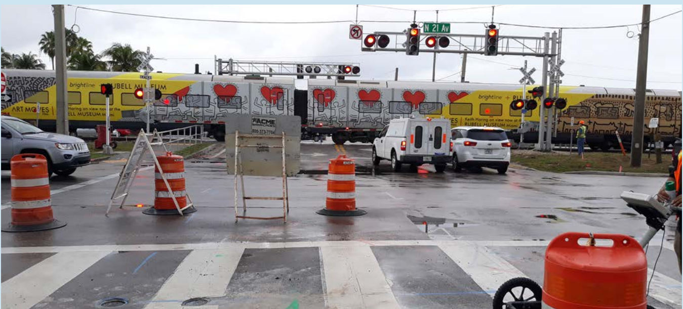
Tetra Tech successfully designed multiple horizontal directional drills of water mains under active railways in Broward County.
