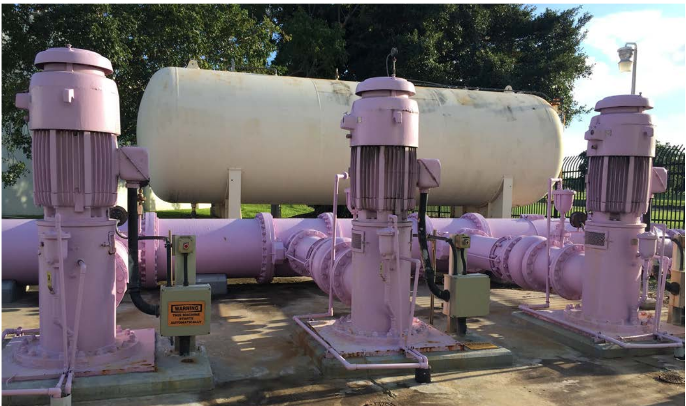
Reclaimed Water Pumps
