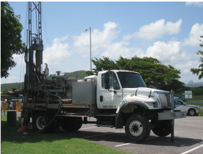
Tetra Tech is a full service engineering firm, with the equipment necessary to implement most projects, including geotechnical engineering.
