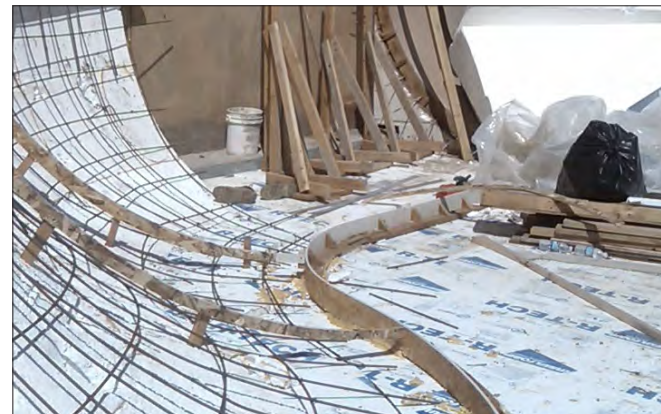
Light-Weight Structural Styrofoam Sub Base Queensborough All-Wheel Park - New Westminster, BC and Seattle Center Skate Plaza - Seattle, WA
