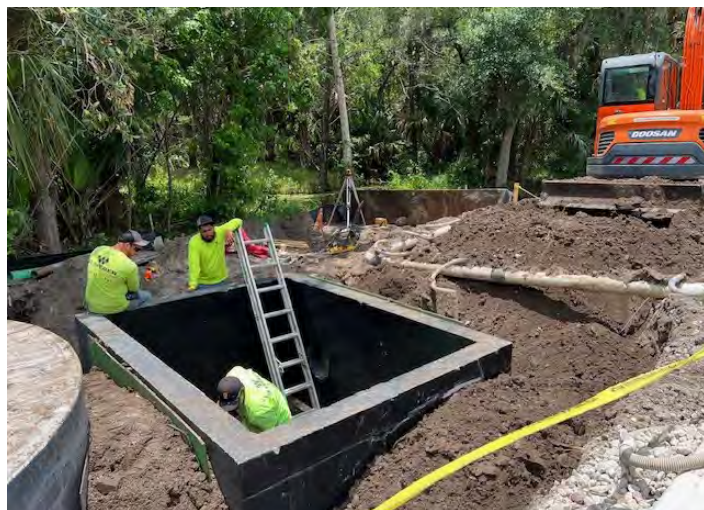
► City of Ormond Beach - Wilmette Ave. Pump Station
