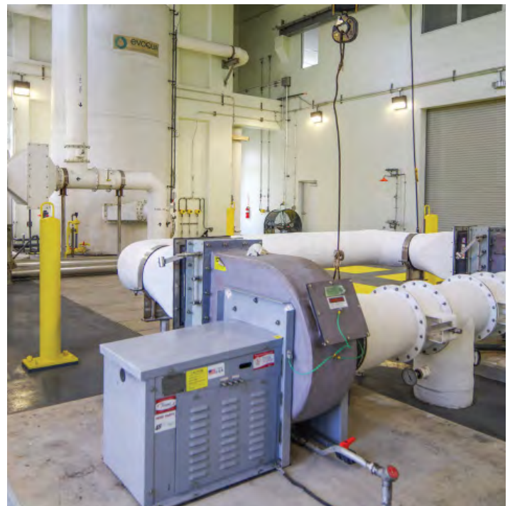
► City of Sarasota - Lift Station No.87
