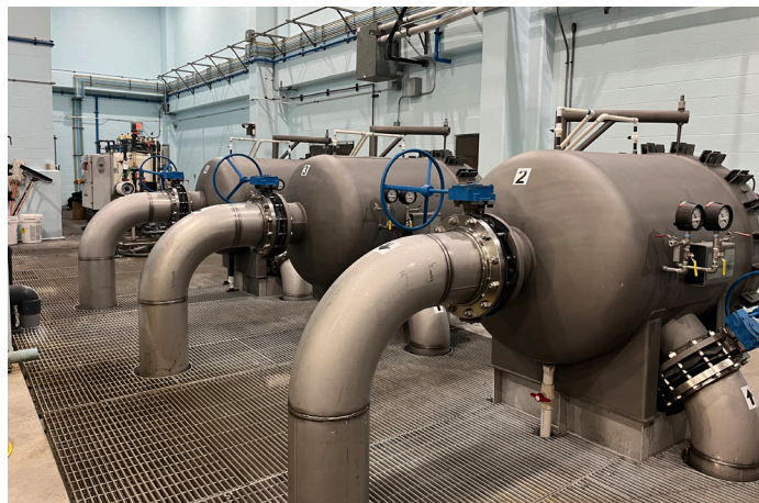
Existing Cartridge Filters at WTP - City of Pompano Beach, FL
