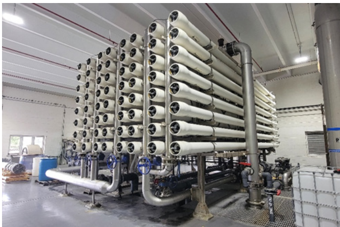
Upsizing of the nanofiltration train and piping - City of Miramar, FL.
