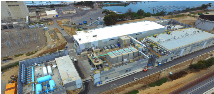
The Carlsbad Desalination Plant (50 MGD) was designed by Arcadis in 2017 and was ACEC National Grand Award Winner.
