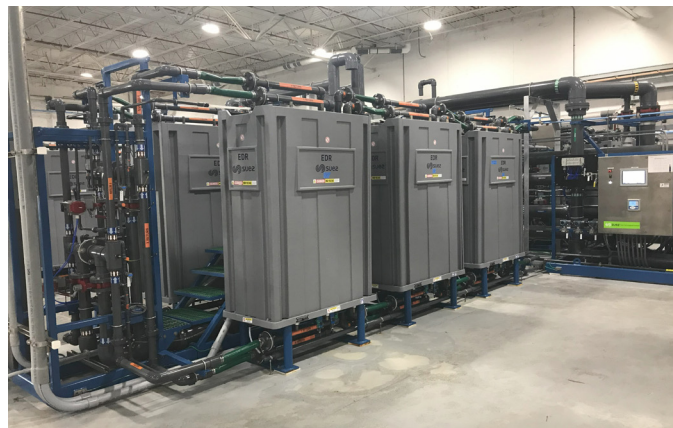
EDR System replaced at Carlton WTP – Sarasota County
