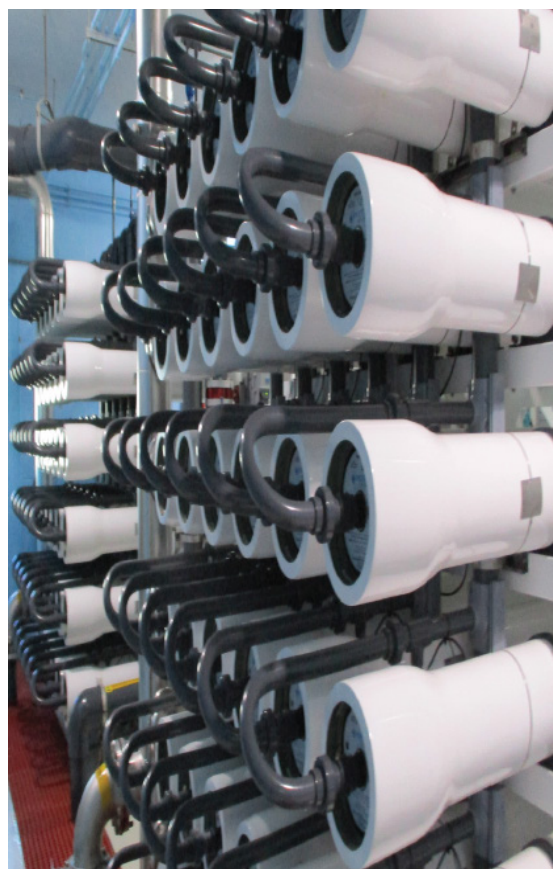
↑ Reverse Osmosis Water Treatment Plant, Venice, FL
