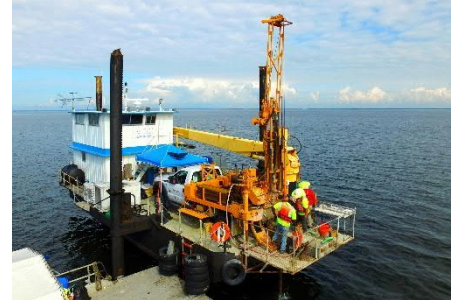
Terracon's Winter Park, Florida exploration team operating a truck-mounted CME-45 drill rig on jack-up boats in Tampa Bay. Borings were performed to depths up to 250-feet- below the mudline to characterize the subsurface for geotechnical parameters.
