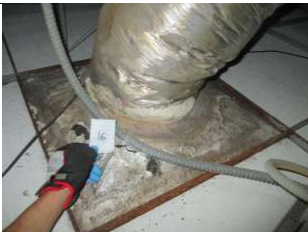
HA 16- White Mastic at Air-Conditioner Vent
