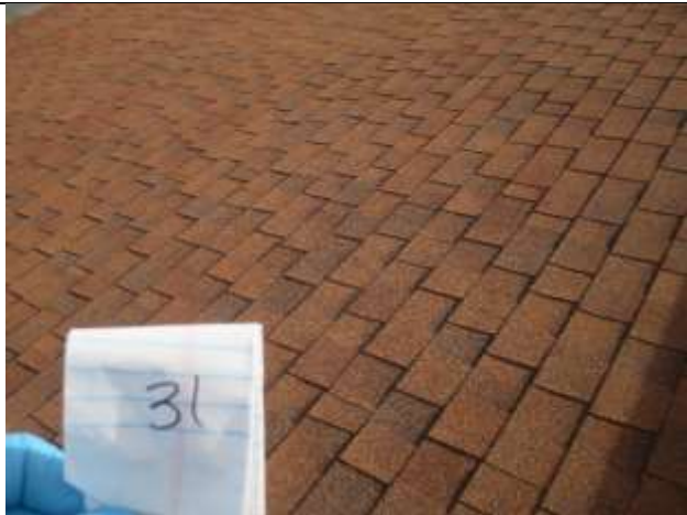
HA 31- Shingles at Roof Sides
