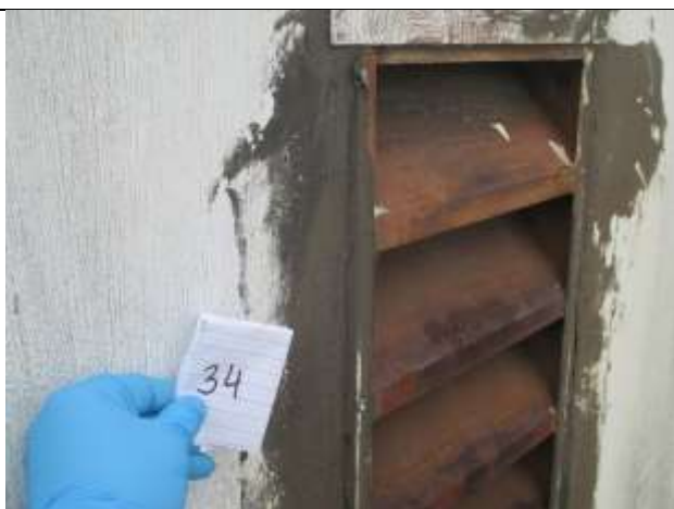
HA 34- Black Mastic at Louvers
