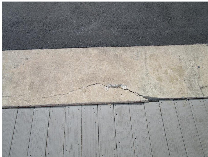
Plate L Significant cracks in concrete cap
