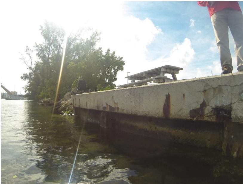
Plate B Southerly View at East End along ICWW. Significant spalling, cracks and staining
