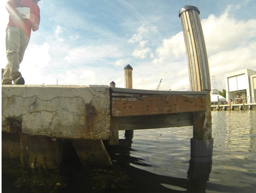
Plate C West View at East End along ICWW. Significant spalling, cracks and staining
