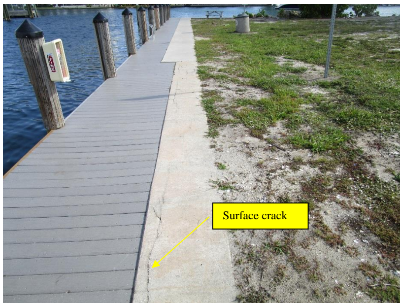
Plate J East view at transition from repaired bulkhead section to original bulkhead structure
