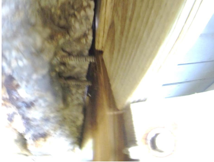
Plate U Severely spalled concrete with evidence that cross member support connections are in poor condition
