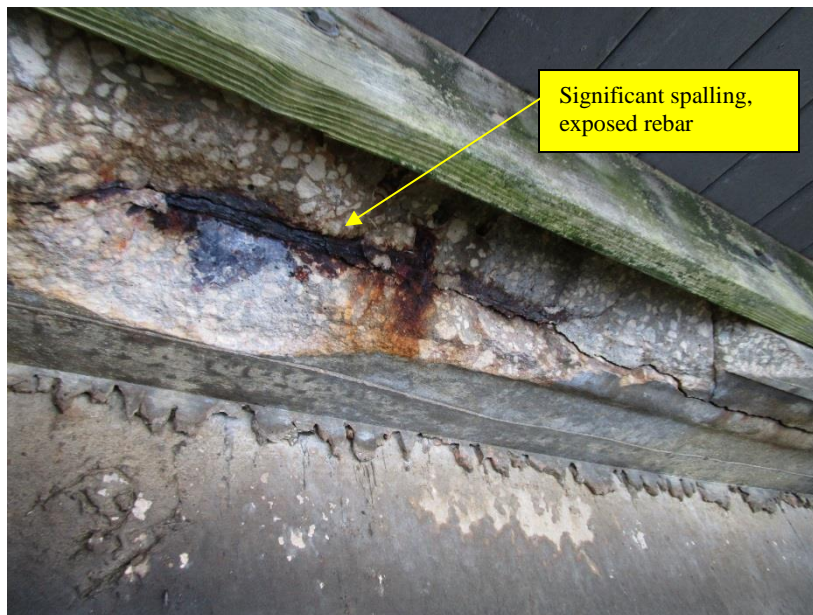
Plate R Typical condition of bulkhead cap
