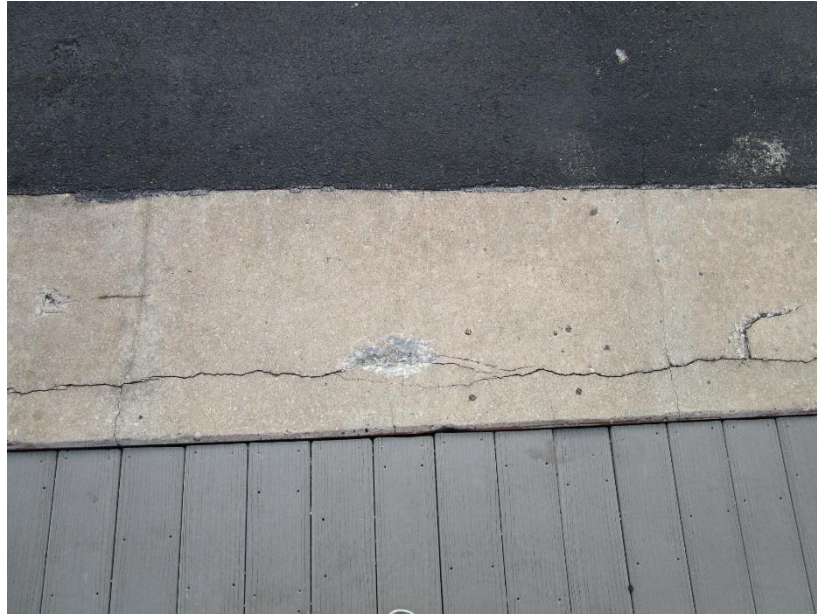
Plate M Significant cracks in concrete cap
