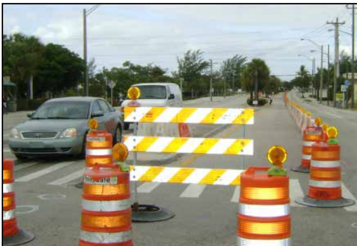
Dr. Martin Luther King Jr. Boulevard Watermain & Streetscape Project Lane Closure for Island Construction
