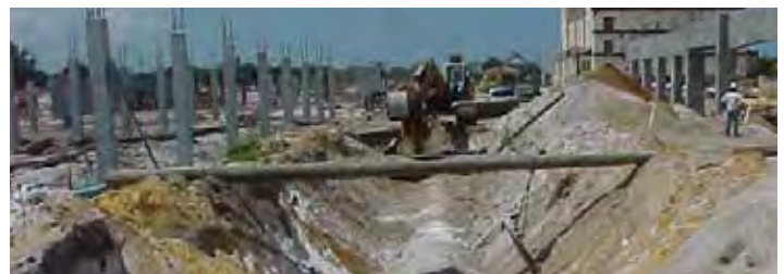
Rosemary Avenue utility relocations underway, while simultaneously constructing the vertical elements of CityPlace.
